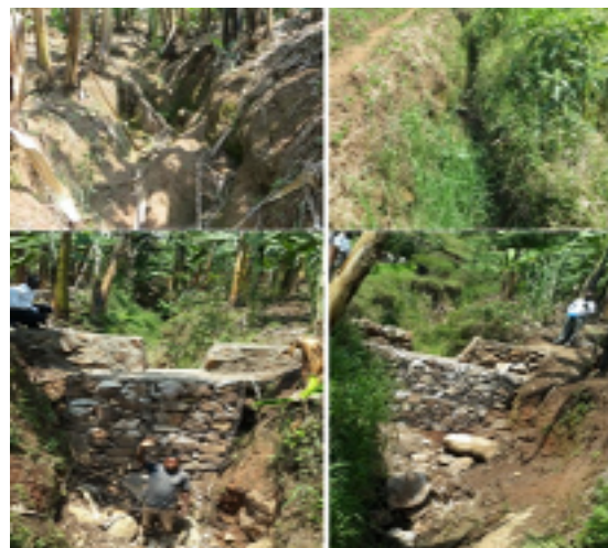
Figure 29: Gullies (Top) and check dams (bottom) constructed in gullies to regulate water flow and to trap debris from upstream
