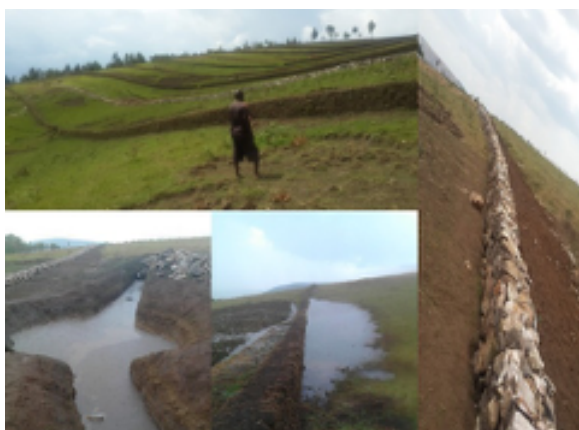
Figure 31: Some of the measures implemented in Mashyoro Micro catchment: stonebunds (top and right) and infiltration pits (bottom left)
