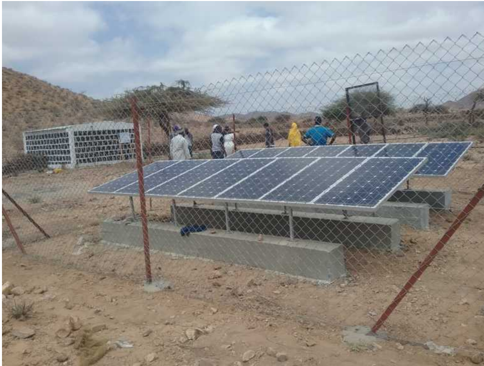
Solar powered pumps
